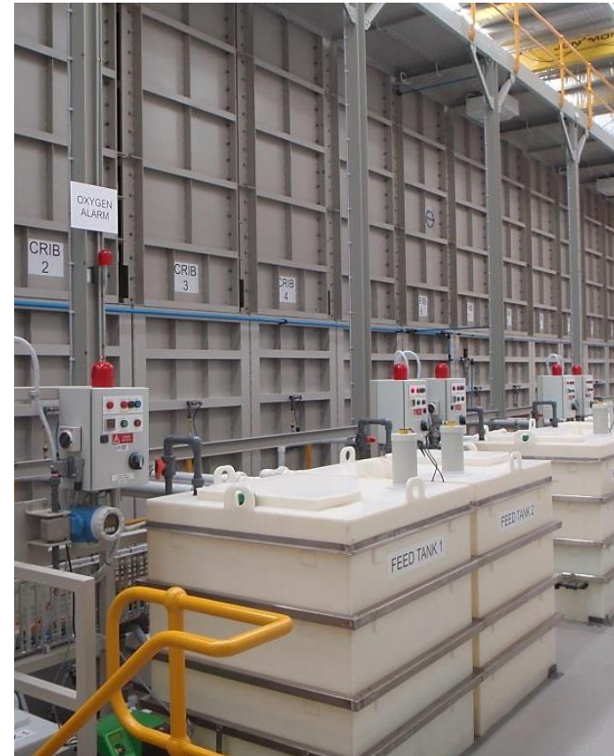
Cribs at heap leach pilot plant facility
